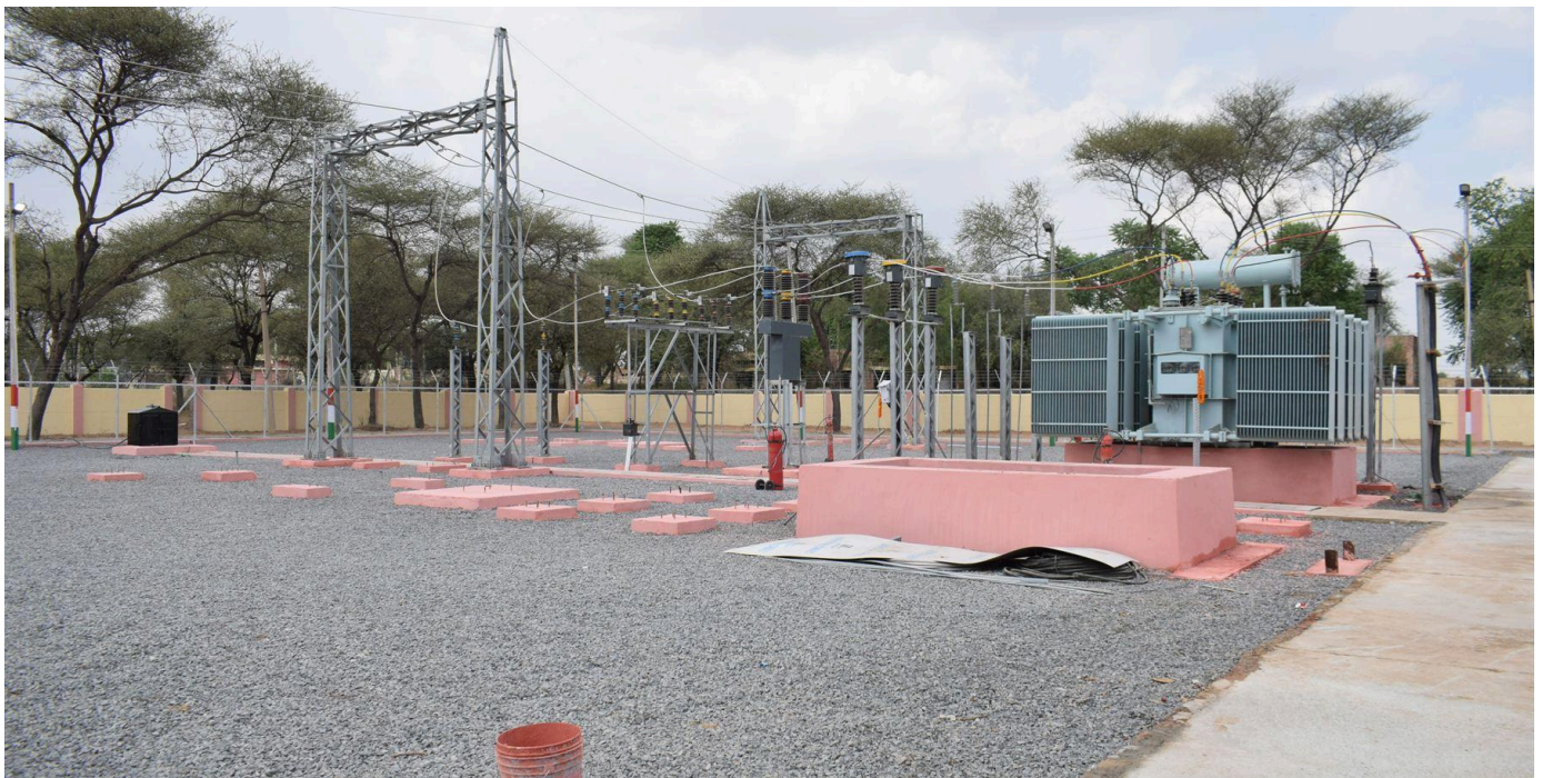
Newly commissioned 33 kV substation, Haryana
